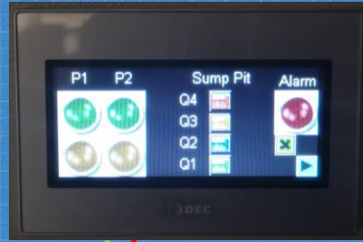
Sump Pump System
