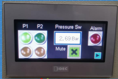
Booster Pump System
